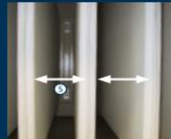
INTERIOR VIEW OF FILTER
