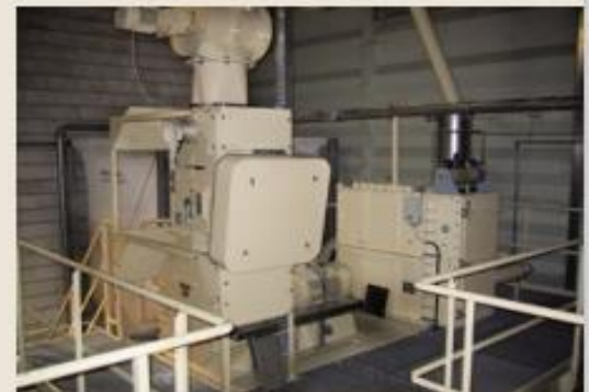
GLECHNER, PFARRKIRCHEN, GERMANY - VL3 ATEX HAMMER MILL DESIGN (ENTRY INTO SERVICE 2003) - WOOD GRINDING: 3 T/H (8 MM FILTER) FOR PELLET PRODUCTION 99% < 4MM
