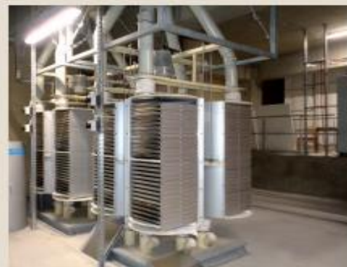
Josera Site in Germany: Preparation of compounds for Petfood. 2 x GDL 20 Module with Plansifter (Grinding concept V3)
