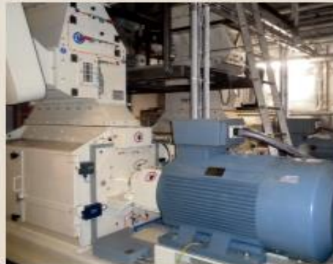
BioMar Site in Denmark: Preparation of compounds for Fishfeed. 2 x VDK 13.1 Module with precrasher
