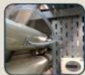
Air flow measurement to control the fan for more energy efficiency
